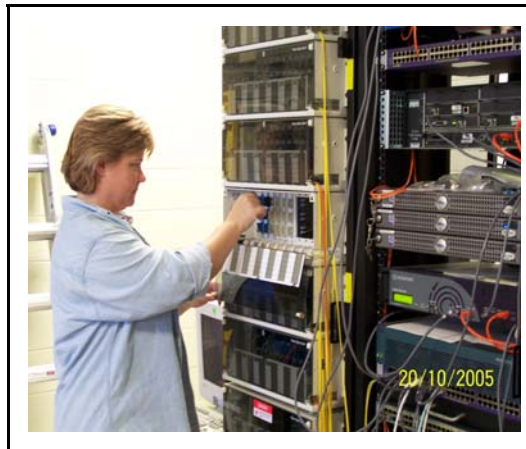
Networking equipment at LSSU
