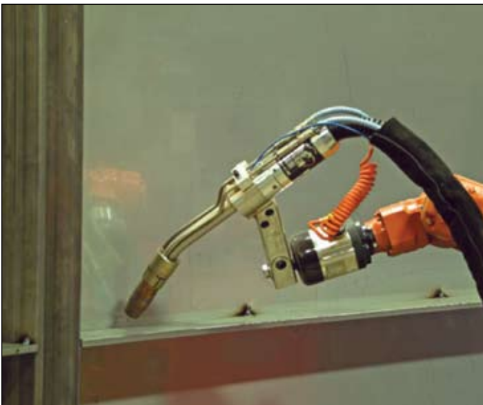
WELDING ON THE SPOT — Robotic welding creates a cleaner, more consistent weld quality and repeatability. It also improve worker safety by preventing employees from being exposed to hazardous welding smoke. (Photo courtesy of VanAire, Inc.)
